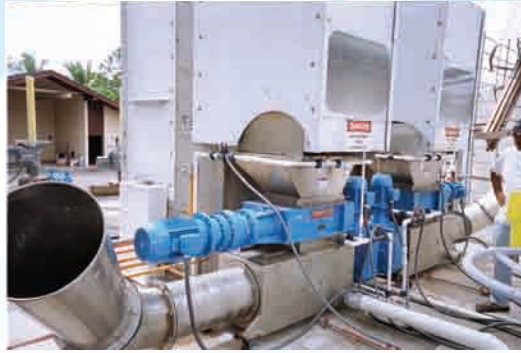
Two SPIRALIFT SC1620 receive screenings from the discharge of two screens.
