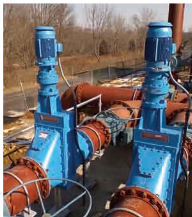
An inline TASKMASTER TM1630 -18 being fed by an 18" force main.
