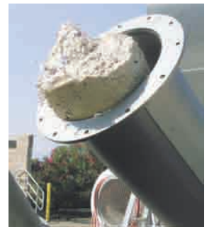
The discharged solids are cleaned and compacted.
